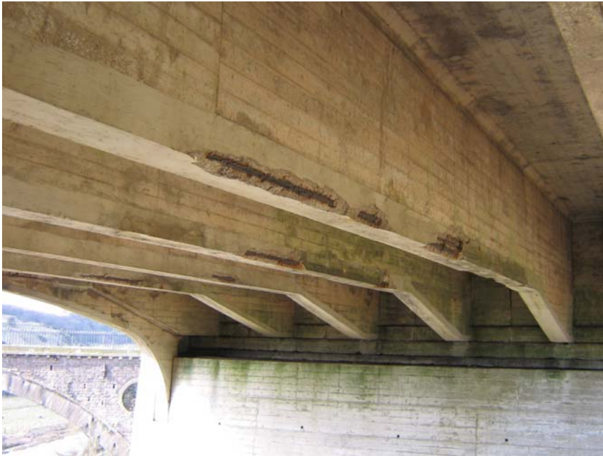
Plate 5: View of support beam disrepair of soffits and arrises
