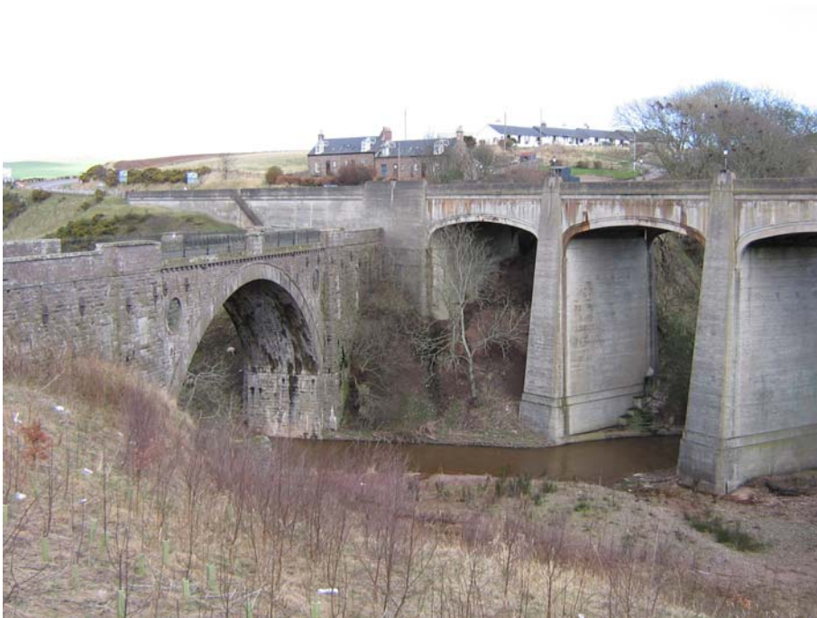
Plate 2: View of second bridge construction dating to 1799 running perpendicular to the Bervie Jubilee Bridge built in 1935.
