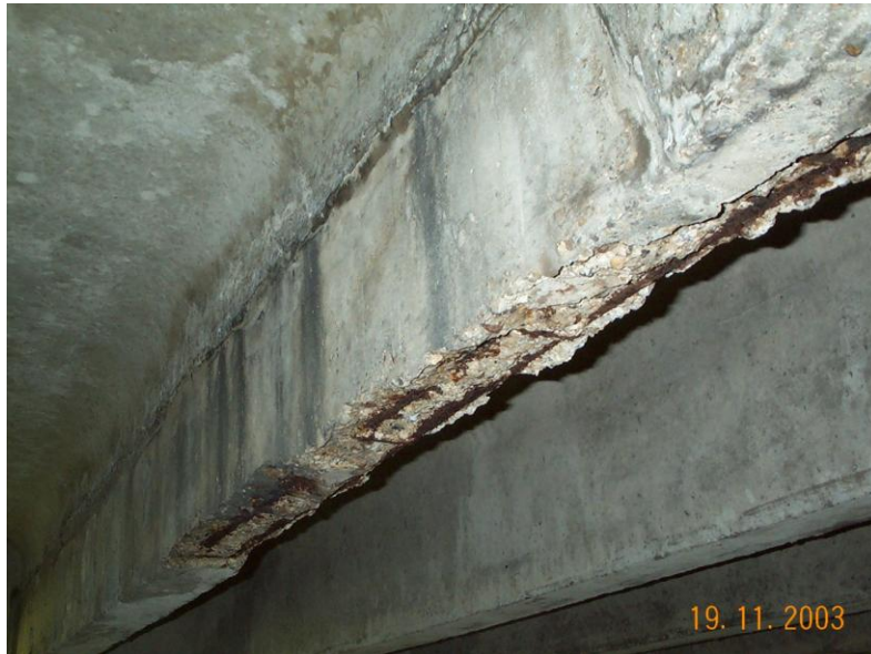
Figure 4: Typical damage to downstand beam arising from leaking chloride-contamination from deicing salts carried in by traffic and through expansion and dayjoints.
