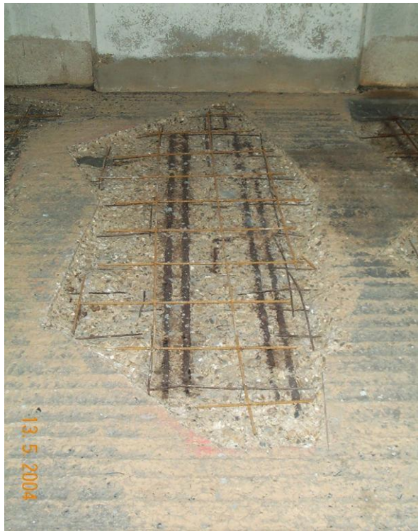
Figure 5: View of reinforcement steel layout and typical corrosion condition with 32mm bars above downstand beams and steel mesh overlaying and spanning to next beam.
