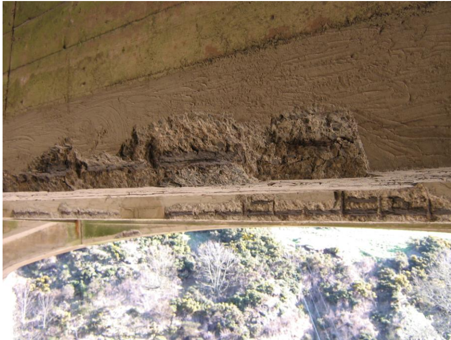
Figure 1: Bridge structure in Scotland showing localised spalling due to chloride contamination; concrete would have fallen some 30m to the ground creating structural, economic and health & safety concerns.
