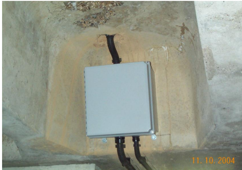
Figure 7: Control and monitoring electronics fitted neatly between downstand beams and protected against damage
