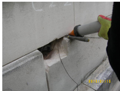
Anode and Wiring Installed Discreetly
