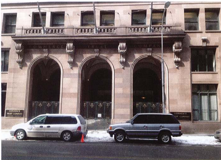
Figure 8: Front entrance of the Commerce Bank in Kansas City following installation of the AACM geopolymer bed joint anode.
