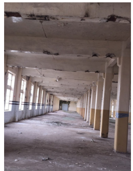
The photos above show the condition and degradation of Terry's before repair and restoration began.
